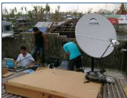
©UNICEF Myanmar/2009 UNICEF IT staff working on the installation of Data Communication network in UNICEF Laputta
