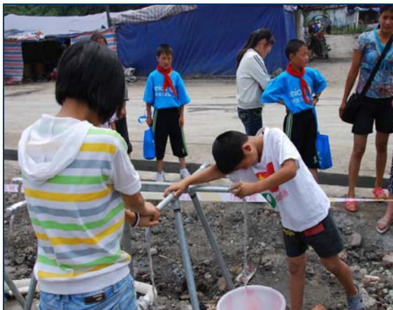
UNICEF provided and helped to install water treatment units to provide safe drinking water to the most heavily-affected areas.
